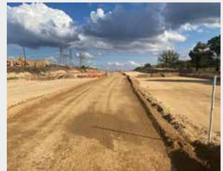
K46 Phase 2 -William Nicol between Juskei River and Diepsloot - Road works in progress
