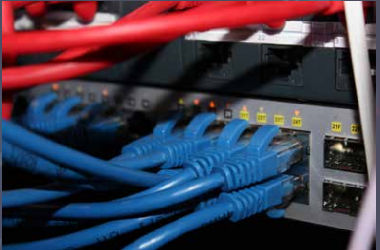
888 sites will be provided with a Wide Area Network this financial year.
